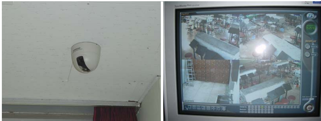
Fig. 5. Surveillance cameras and multi-fractioned monitors.
