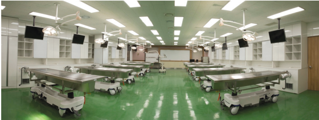
Fig. 2. Panorama image of the anatomy laboratory equipped dissecting tables with inbuilt exhaust and an air diffuser/return system.
