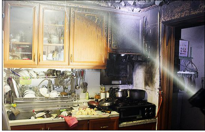
<Fig 13> Kitchen Images where the Fire Took Place.
