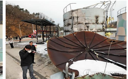
<Fig 8> Roof of Exploded Outdoor Storage Tank.
