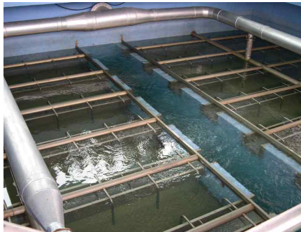
<Fig 1> A Filtration Basin of Water Treatment Plant
