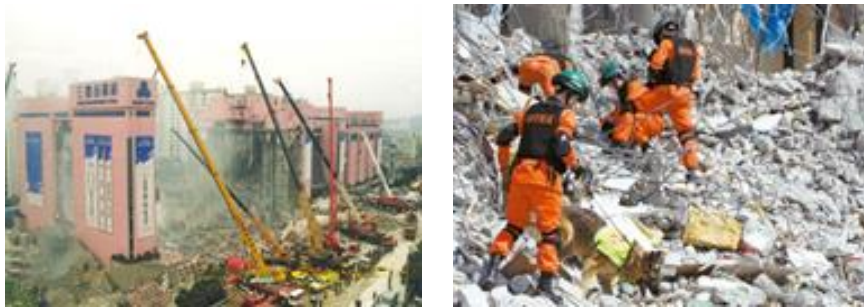
(a) Previous relief method (Remove debris from the top using heavy equipment and manpower)
