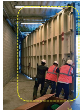
Figure 12. Loading dock type flood gate
