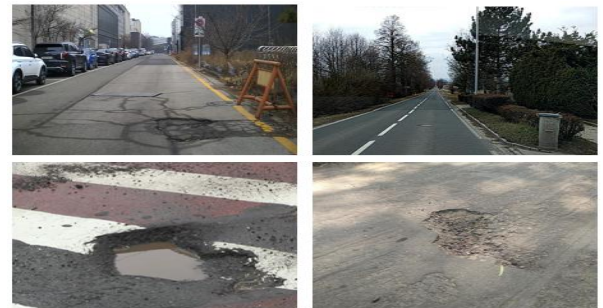
Fig. 5. Examples of Pothole Class
