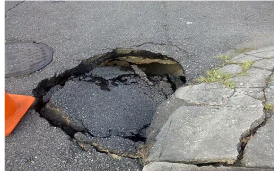
Fig. 1. Example of a Pothole
