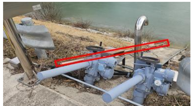
Fig. 9. Water level gauge installed in a reservoir
