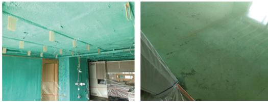
Figure 3. Example of application of the shielding method to reduce indoor radon in Daejeon Metropolitan City.
