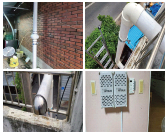
Figure 2. Example of application of the soil ventilation method to reduce indoor radon in Daejeon Metropolitan City.
