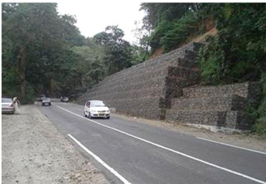
Figure 8. Examples of Slope Stability Measures for NH 516E Paderu-Araku Road Section (Ministry of Road Transport and Highways, Government of India, 2019)
