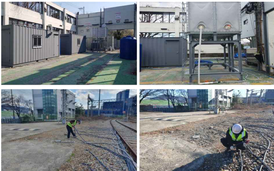
Figure 5. Installation and operation of soil flushing facility
