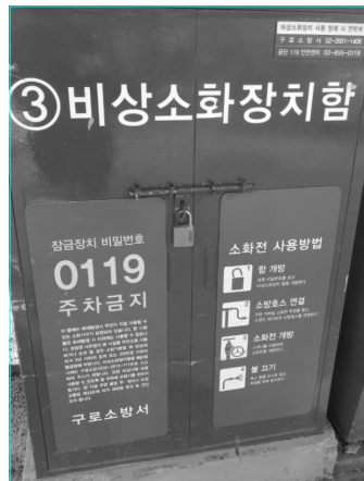
Figure 16. Emergency fire fighting equipment box(비상소화장치함) in front of Garibong-dong community center and Guro-gu Happy Family Support Center
